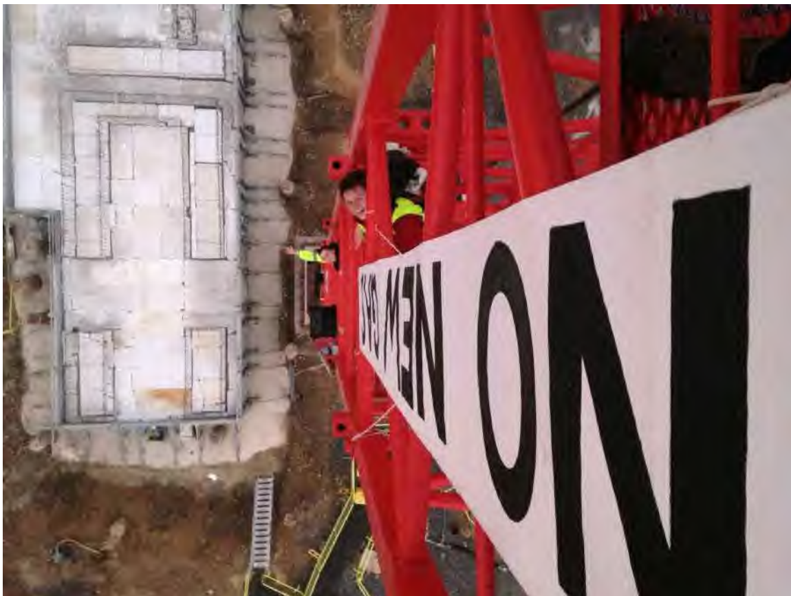
Activists spent 15 hours occupying a crane and blockading the entrance to the UK's only gas site currently in construction, shutting down operations for the day in Keadby and taking over regional news with our message: Gas ain't green!
