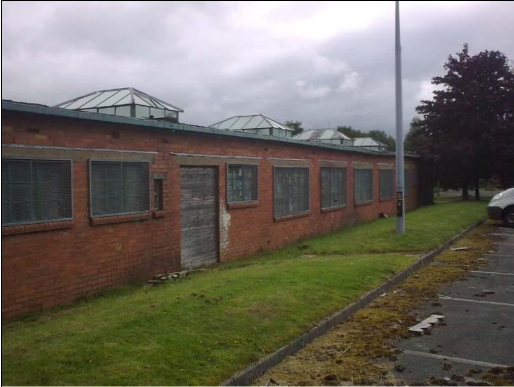
Plate 5: building at TN12 in the southern section of the site with moderate bat roosting potential
