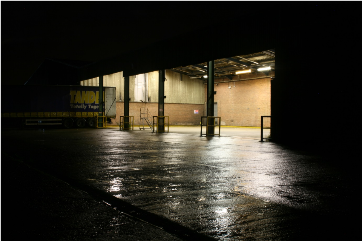
Figure 0.15: Type D lights on north side of Building (Service Yard).
