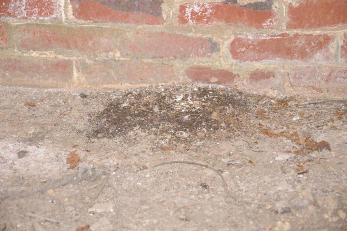
Photograph 11: Building 8 – droppings in tower.
